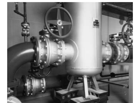
City Gas piping around governor
