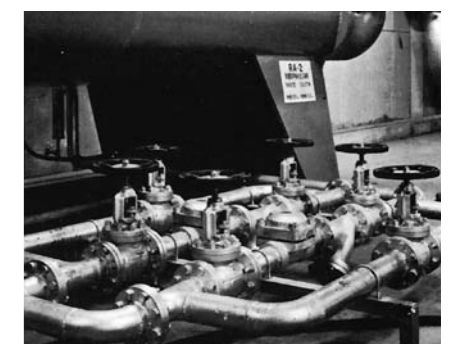
Piping around freezer
