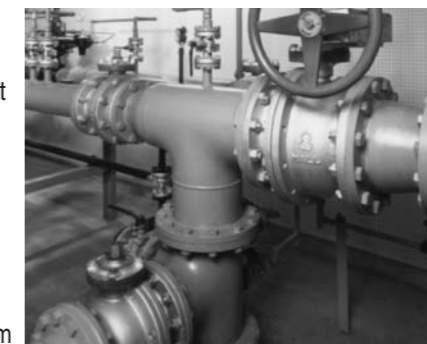
City Gas piping around governor
