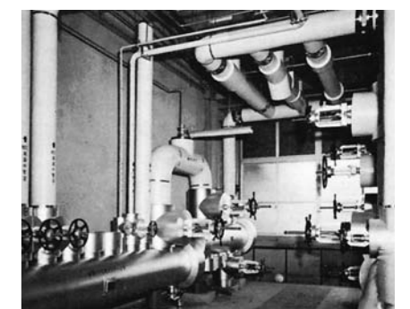
Hot water line
