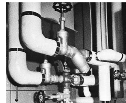
Hot water line
